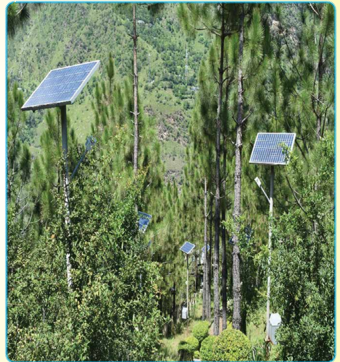
Independent Solar LED Light at Jhakri
