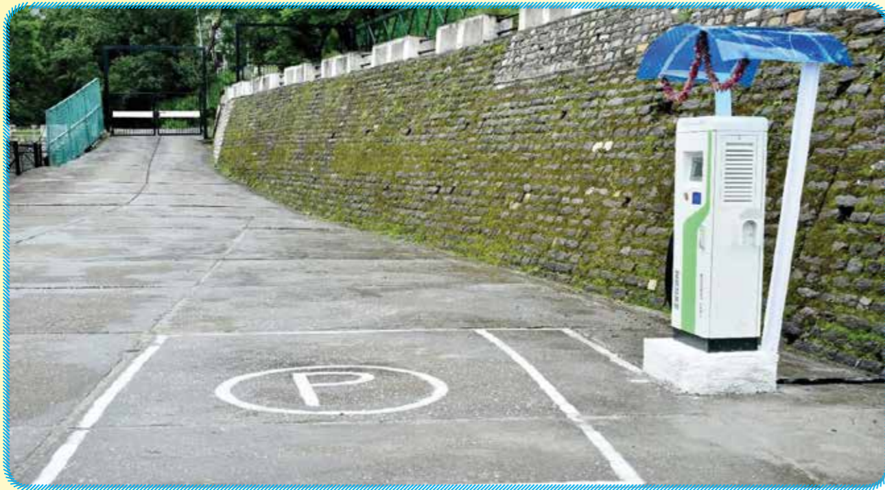
Electrical Charger for Charging of Electrical Vehicles
