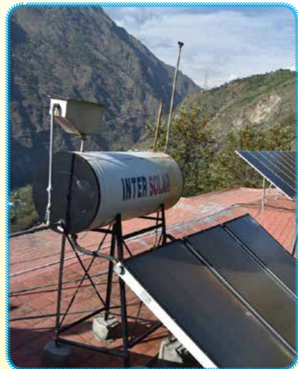
Solar Water Heater Plant at Main Administrative Building
