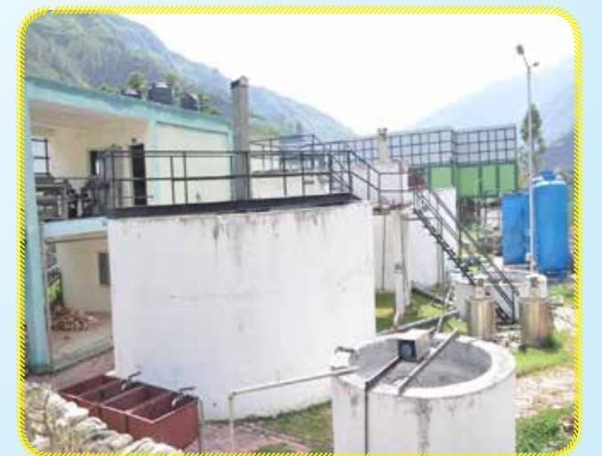
STP of 400 KLD at RHPS
