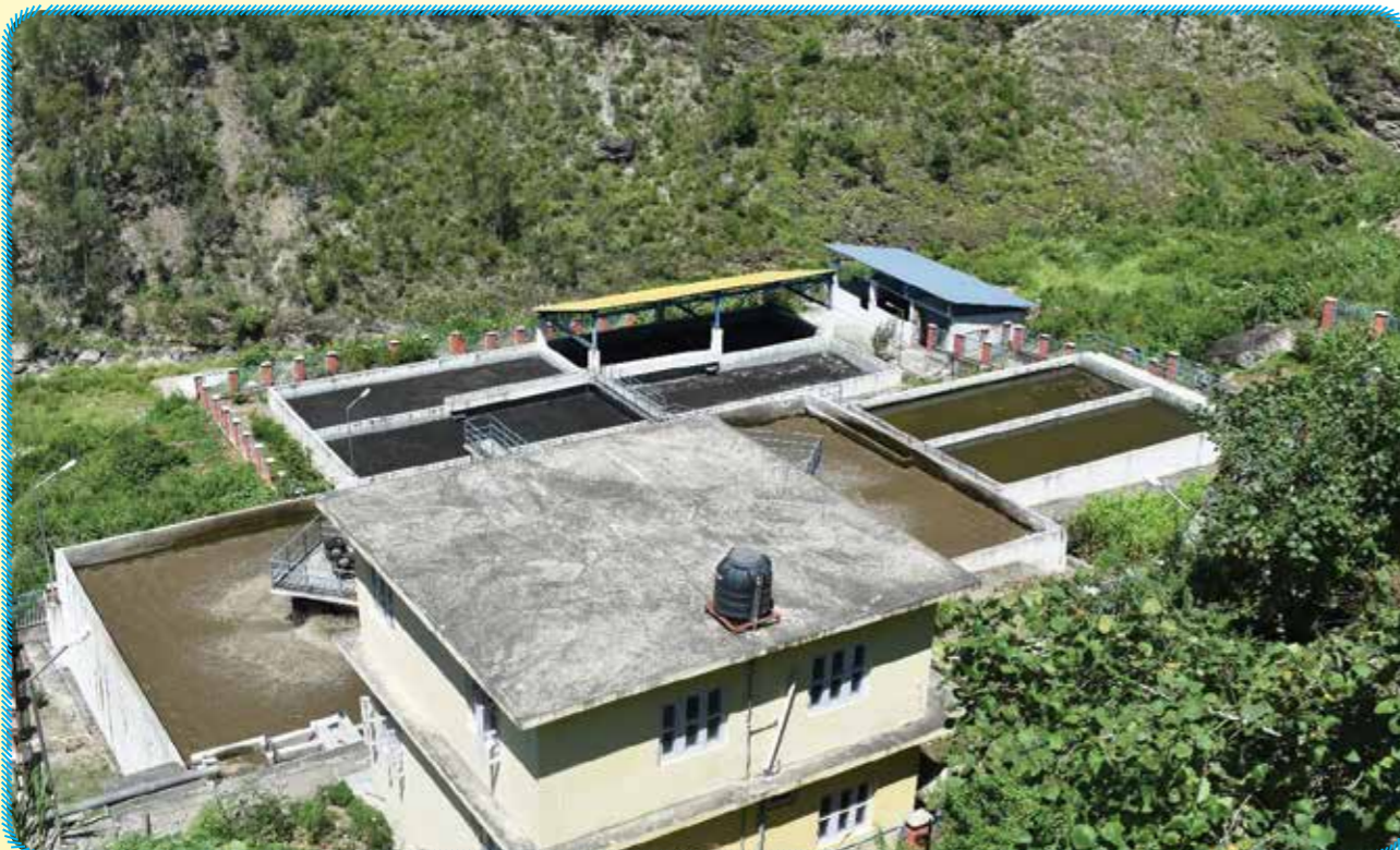
Sewerage Treatment Plant to cater to Village Jhakri
