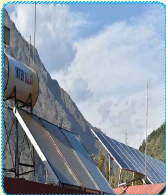
Solar Water heaters at Mayur Bhawan Guest House
