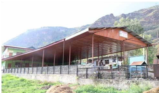
Construction of roof on open space in front of Community Centre, Bayal, Gram Panchayat Gadej, Tehsil Nirmand, Distt. Kullu, (H.P)
