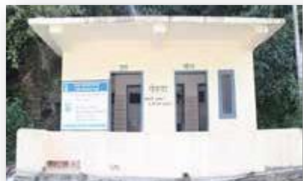
Construction of Toilet in village Brow, Gram Panchayat Brow, Tehsil Nirmand, Distt. Kullu (H.P.)
