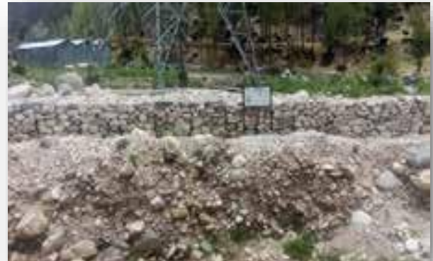
Diversion of Nallah to original course and protection work at village Bainol as safety/relief measure of cloudburst
