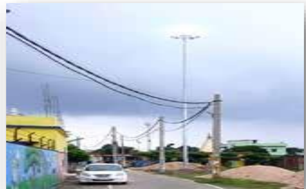
Installation of High Mast Light at Chipura Gram Panchayat, Smapatchak, Patna, Bihar
