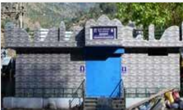
Construction of Public toilet at Chaudhary Adda (Old bus stand), Rampur, H.P.
