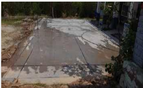
Construction of Badminton Court in Govt Primary Sec. School Lehri Sarel, Distt. Bilaspur (HP)
