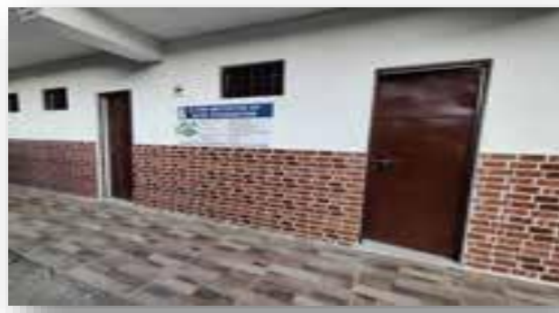
Construction of toilets at Govt. Sr. Sec. School, Pujarli-4, Distt. Shimla, H.P.
