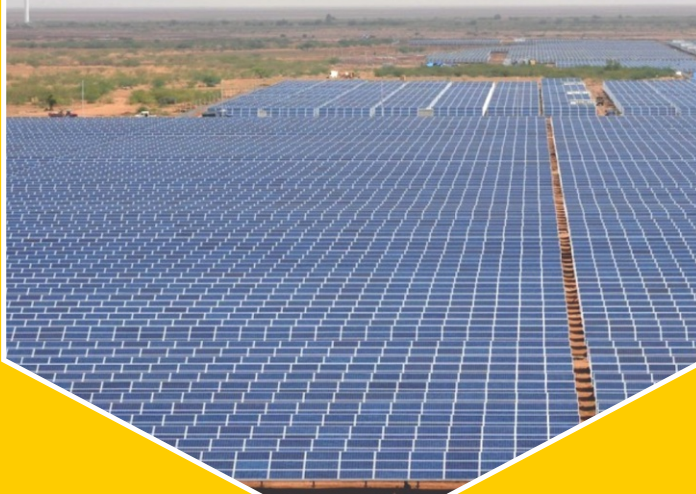
5.6 MW Solar Plant at Charanka Solar Park, Gujarat
