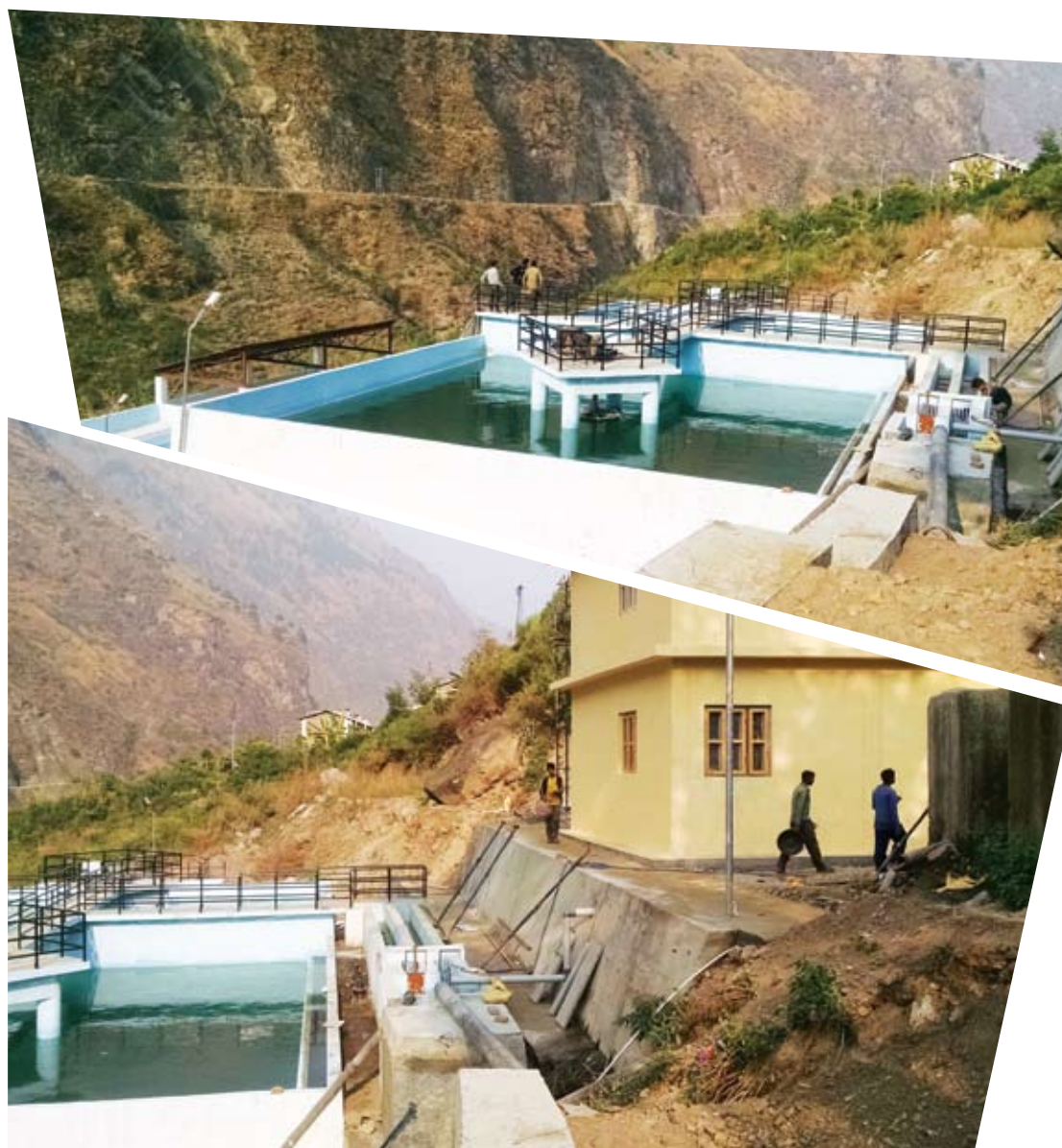
Sewerage treatment plant at Jhakri
