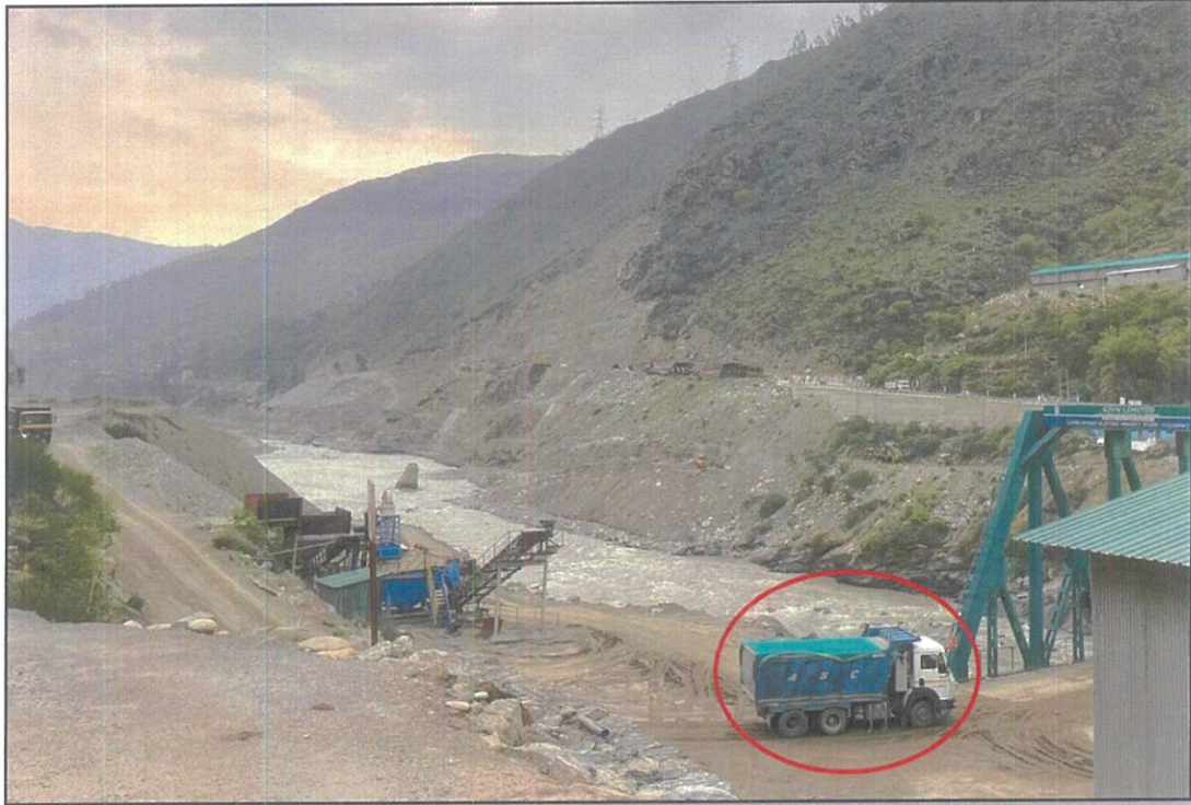
Dumper covered with net to avoid dust emission & Water sprinkling at Dumping yard.
