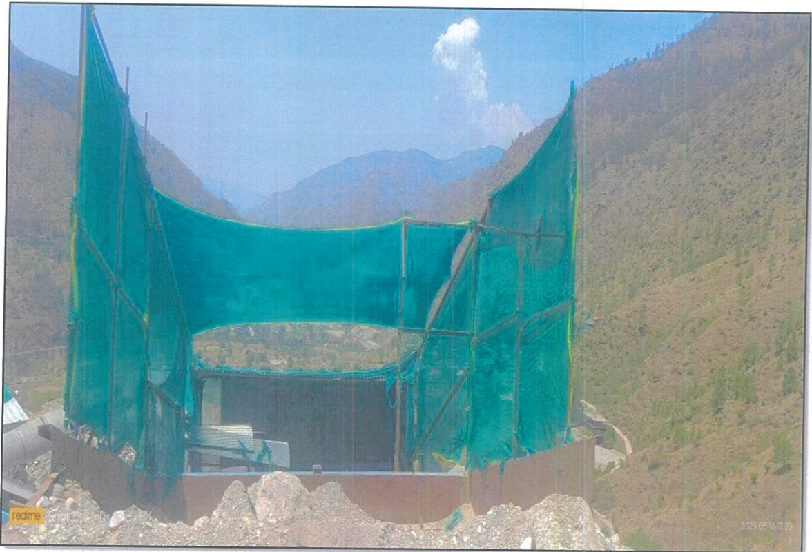
Picture-6. Crusher parts properly covered to prevent dust emission.
