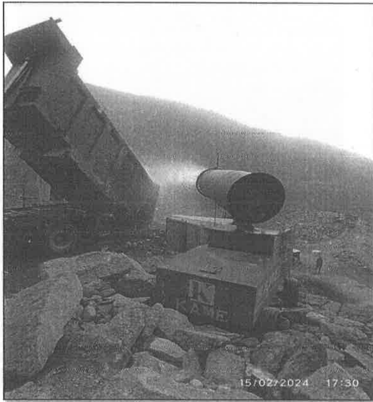
Picture-2. Water sprinkler being used at Crusher Plant.
