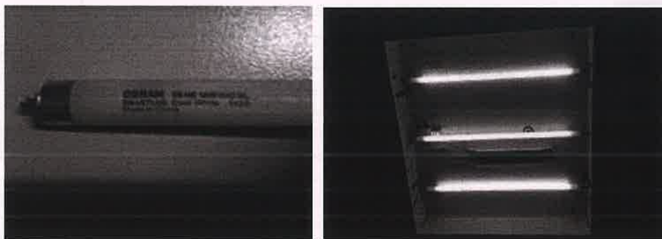
Conventional T-5 FLT Recessed Mounted Light Fixtures with choke installed in SJVN
