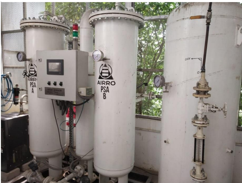
Figure 70: Oxygen Plant installed in Himachal Pradesh
