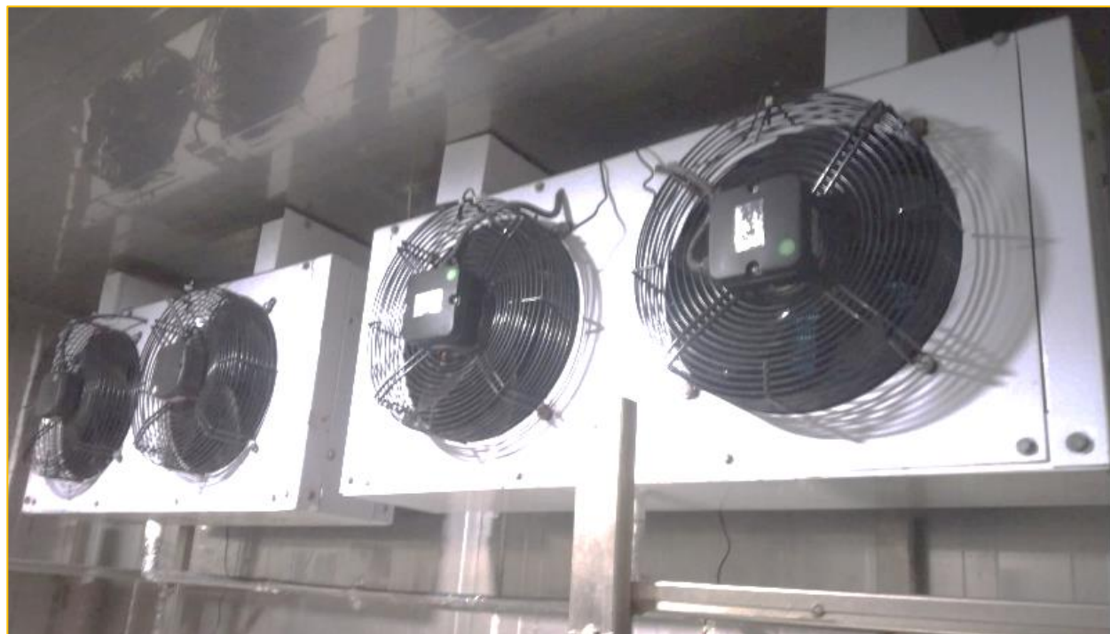
Figure 38: AC vents at the cold chain
