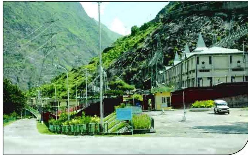
Power Transmission - Pot Head Yard (NJHPS)
