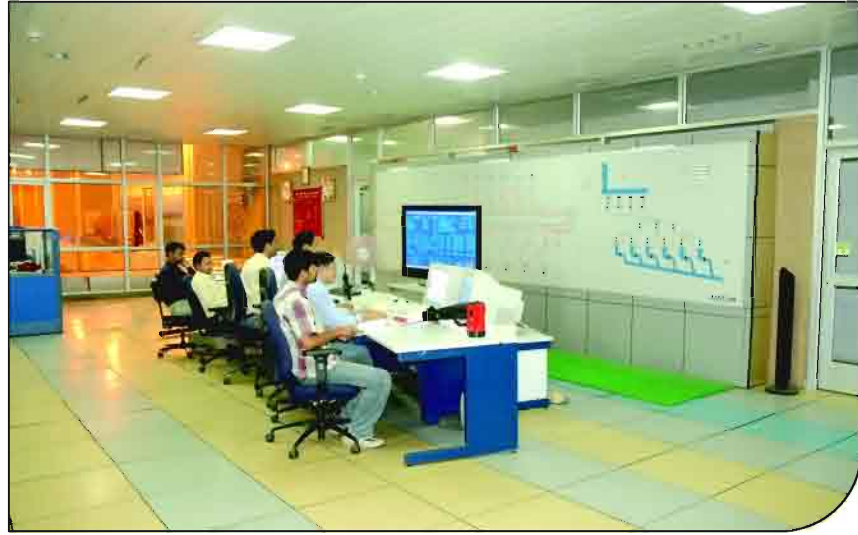
Power House Control Room
